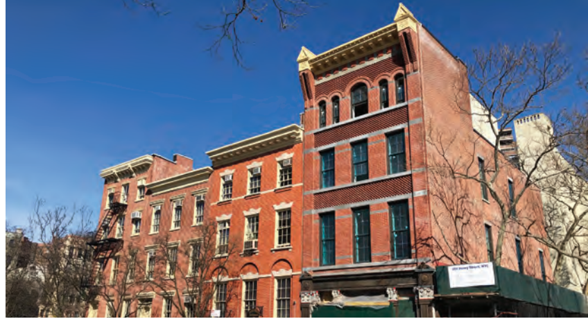
Construction is nearly complete on the historic three-story firehouse at Henry Street Settlement
